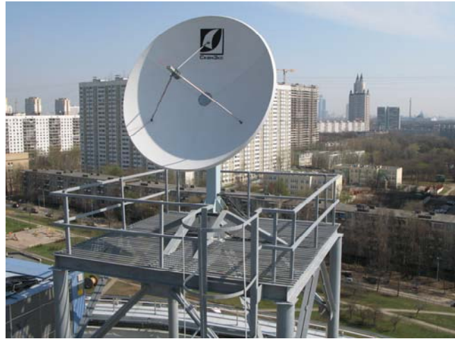
UniScan hardware and software complex installed at National Centre for Crisis Management
